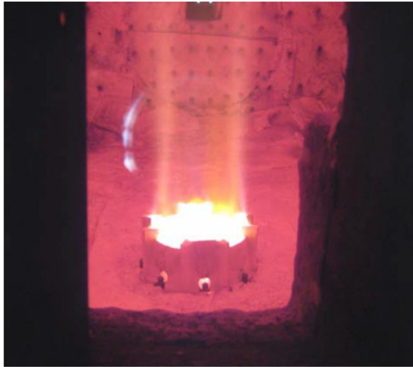
Figure 3: Hydrogen Combustion in Industrial Burner Test 60
