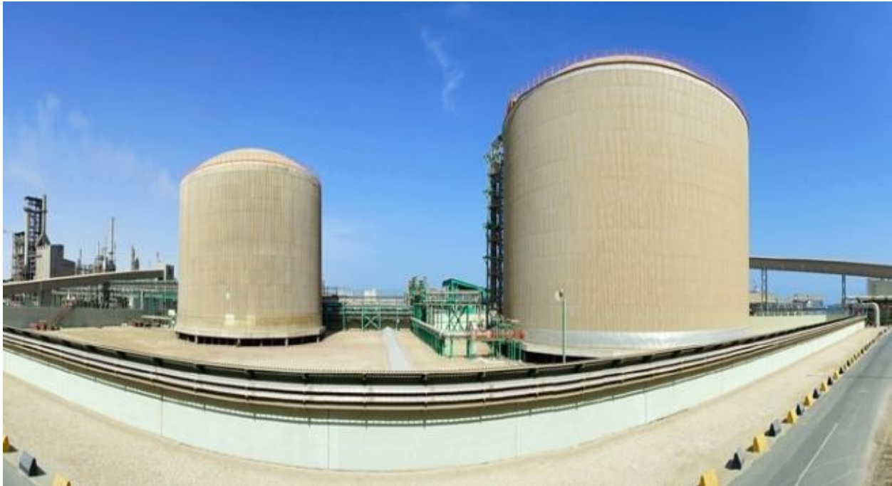
Fig. 5. QAFCO Ammonia Storage Tanks - Messaieed, Qatar
