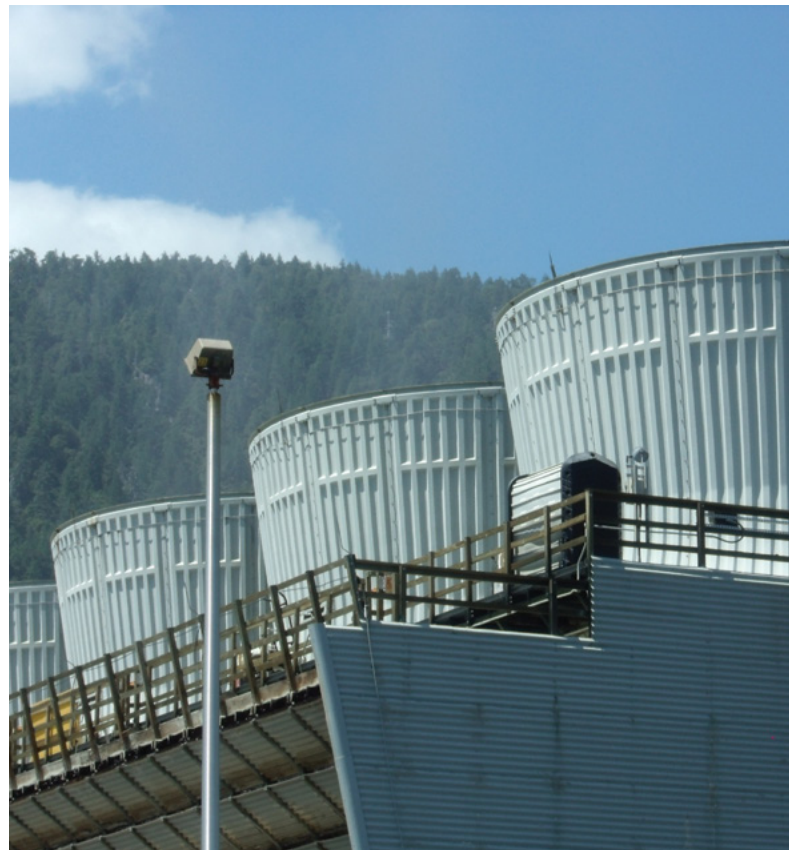
An evaporative cooling tower at Socrates Geothermal Power Plant (The Geysers, California). Photo credit: Geothermal Resources Council
