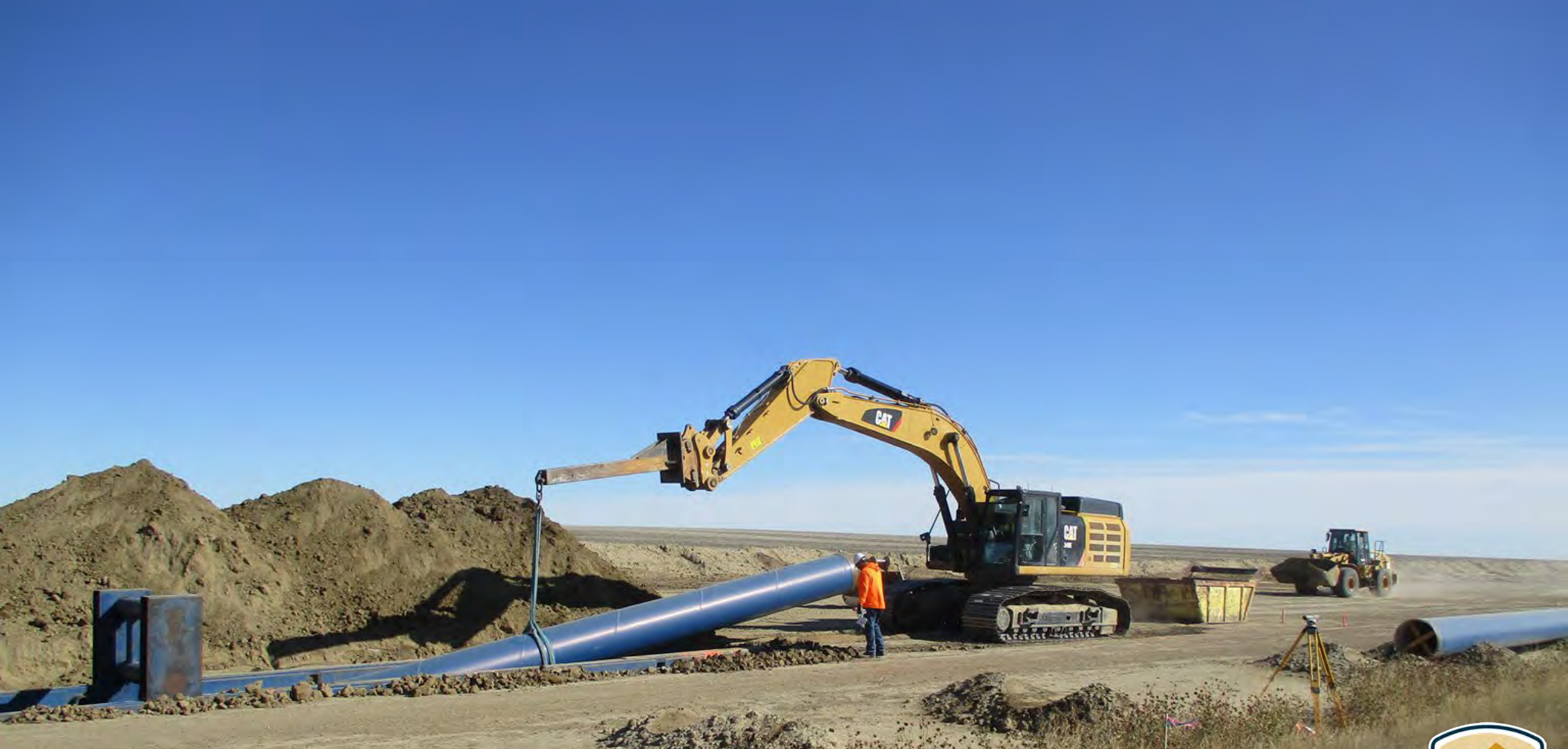
Rocky Boys Rural Water Project Construction, Montana $58M in BIL funding in 2022 and $78M in 2023
