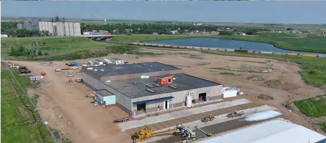
North Dakota Rural Water Construction $77 million in BIL Funding, including Tribal construction programs, including the Northwest Area Water Supply Project
