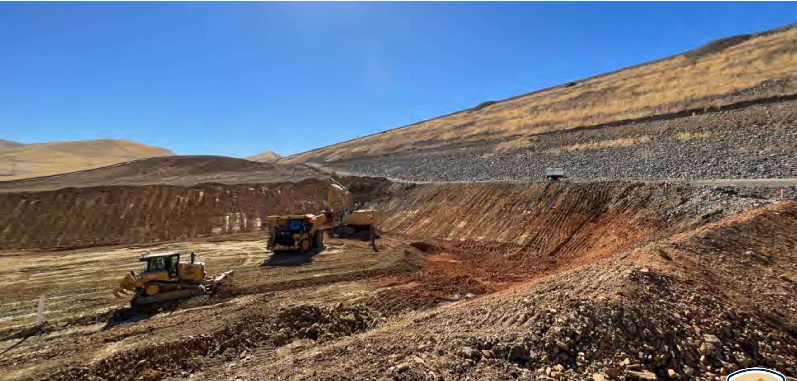
B.F. Sisk Dam and San Luis Reservoir Heavy Machinery Excavating Slope California, November 2022 – $100M in BIL funding in 2022
