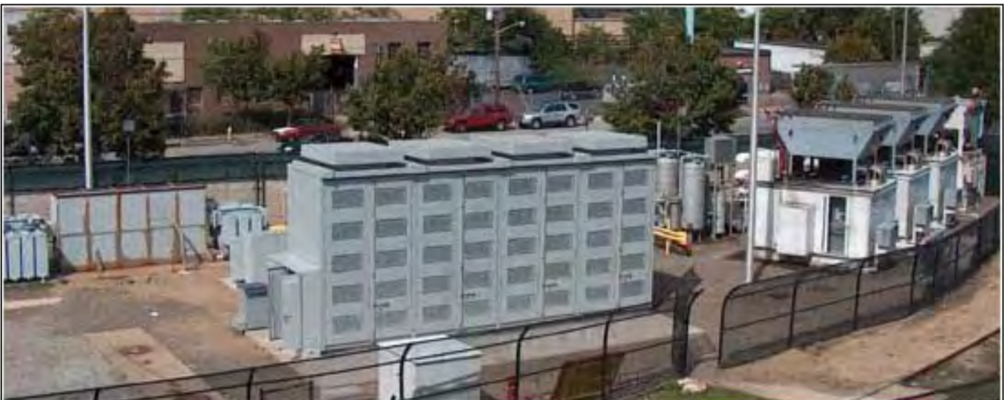
Sandia National Laboratories advanced sodium-sulfur battery energy storage system
