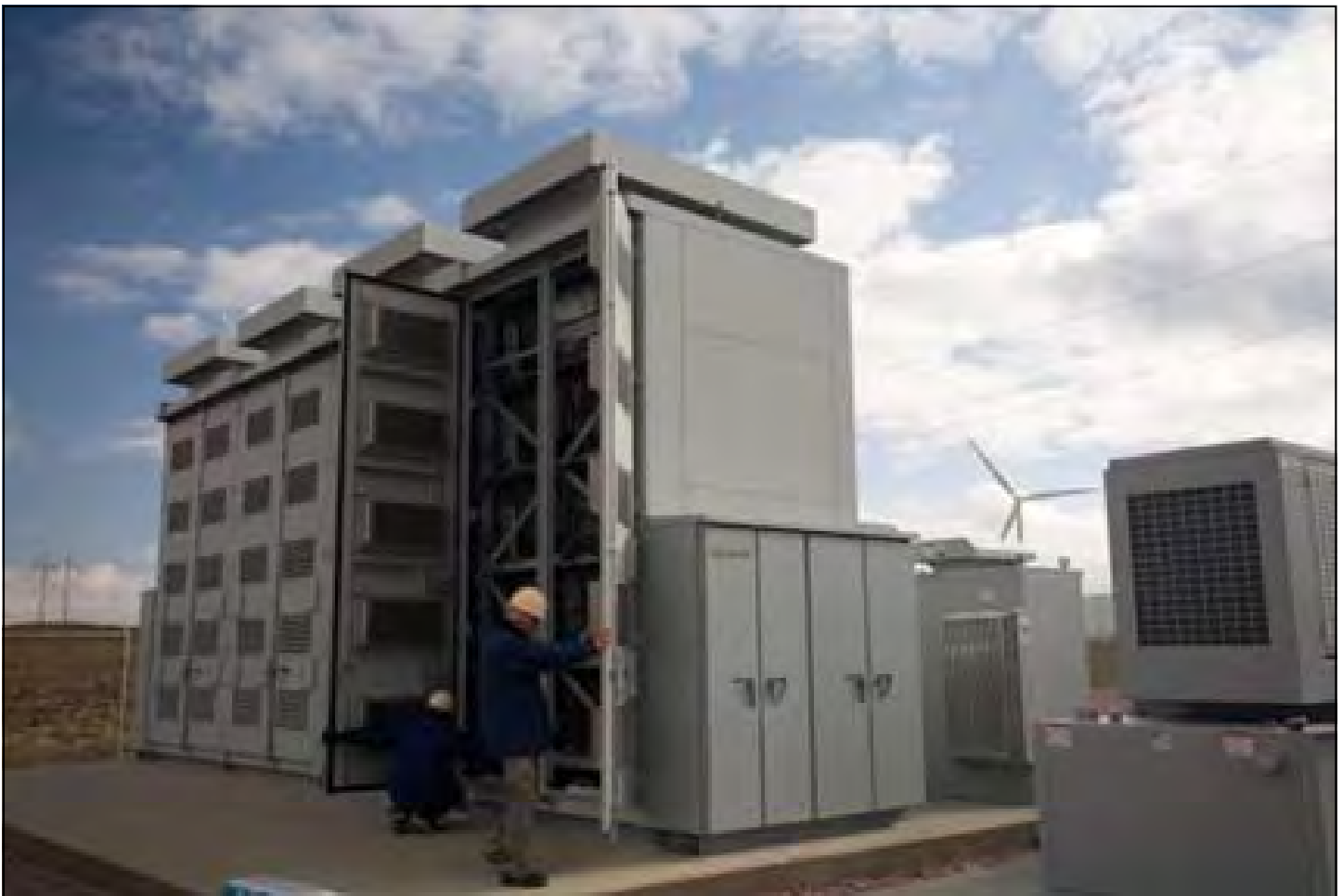
Xcel Energy wind-to-battery project, Minnesota
