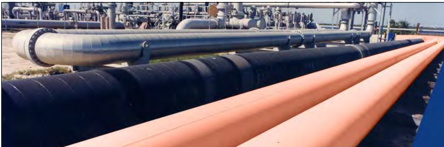
Strategic Petroleum Reserve crude oil pipelines, Bryan Mound, Texas
