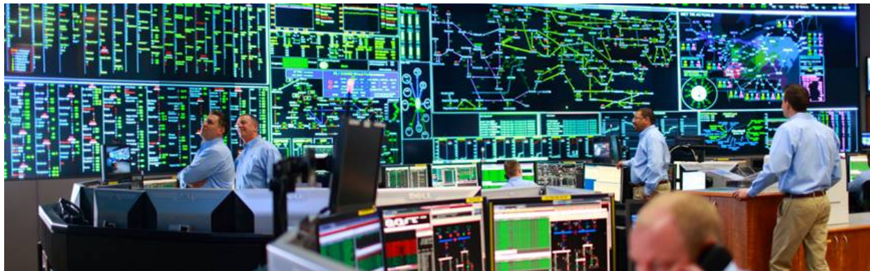
Figure 6. System Operations – PJM Control Room
